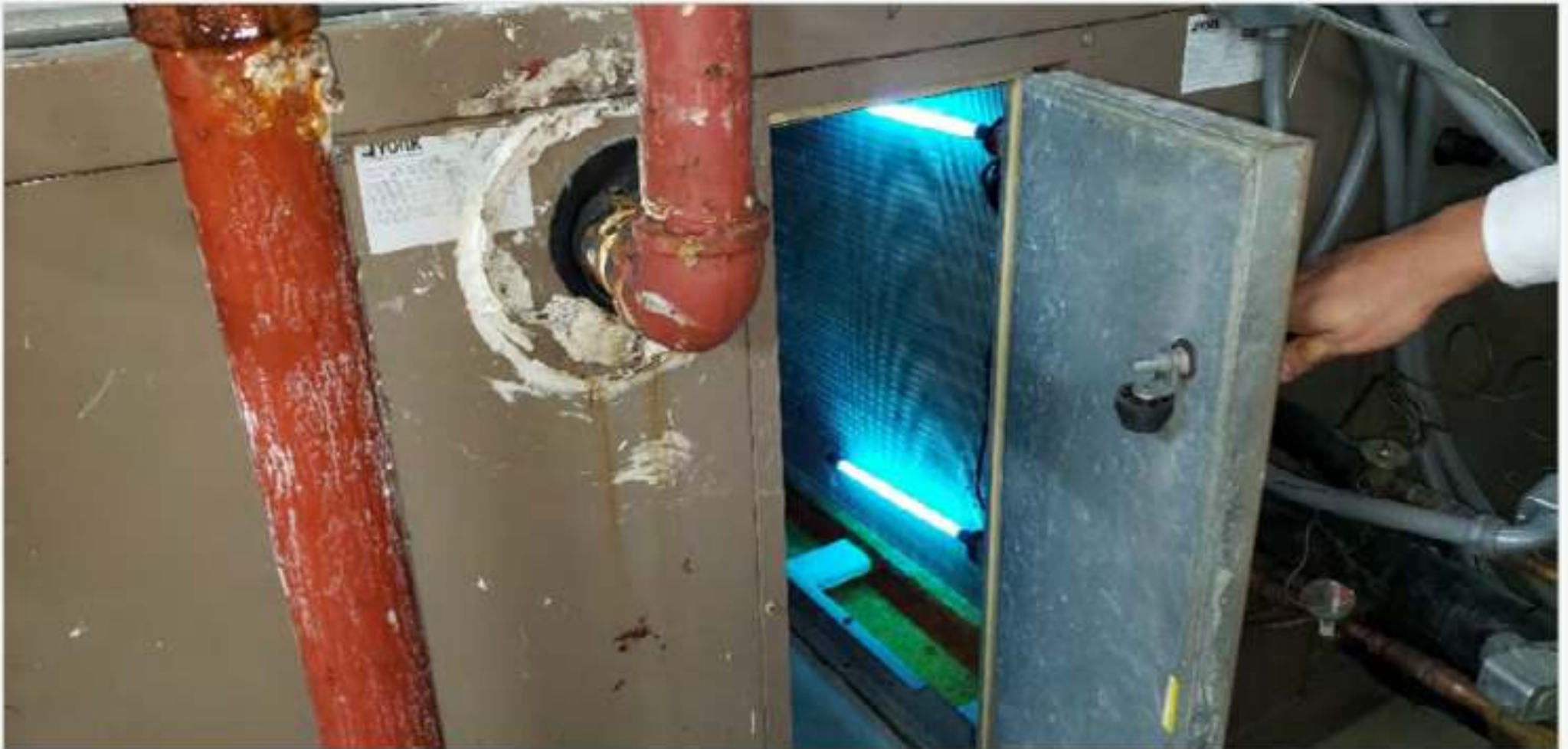
Figure 9. UVGI lamps installed upstream of the cooling coil
